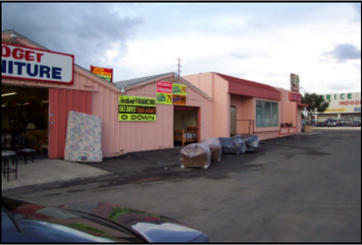
Photo 4: These commercial buildings are improperly used for retail sales. The buildings are built of corrugated metal and designed for warehousing uses. The site also lacks landscaping and pavement.
